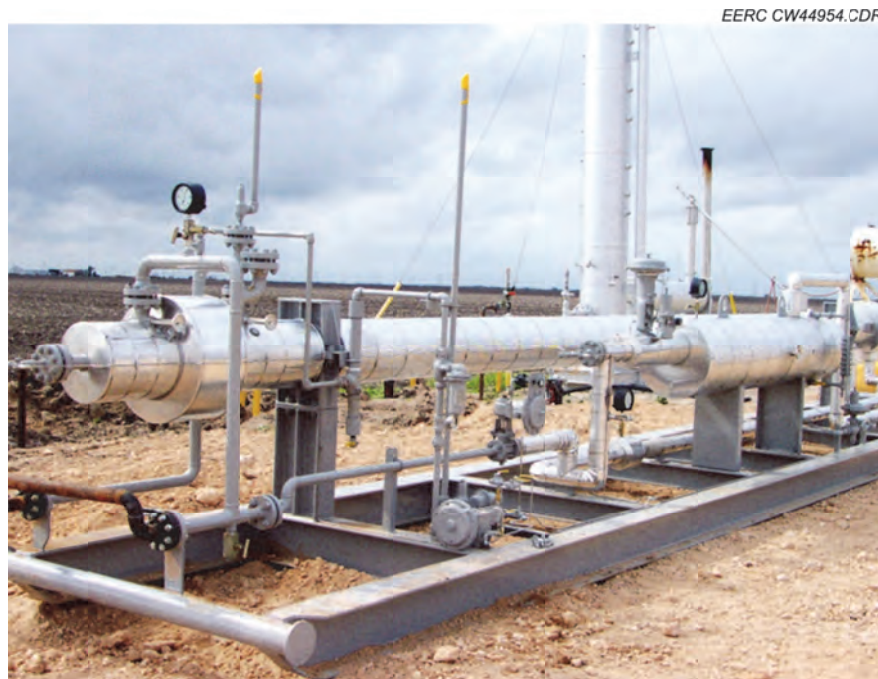
Figure 49. Small JT NGL recovery skid as provided by dew point control.
