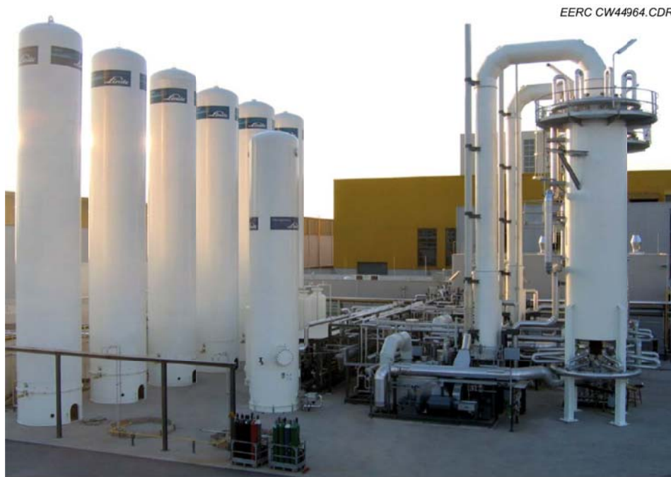
Figure B-3. Approximate 300-lb/hour SMR hydrogen production–purification unit.
