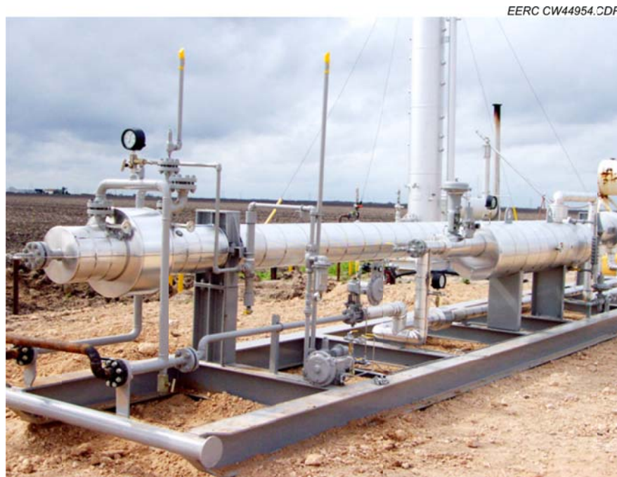
Figure 20. Small JT NGL recovery skid as provided by dew point control.
